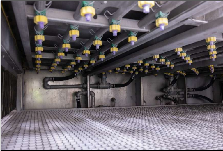
Interior of spray zone
