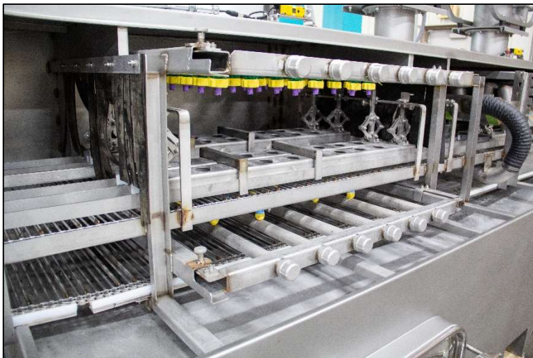
Interior of four-lane cleaning system
